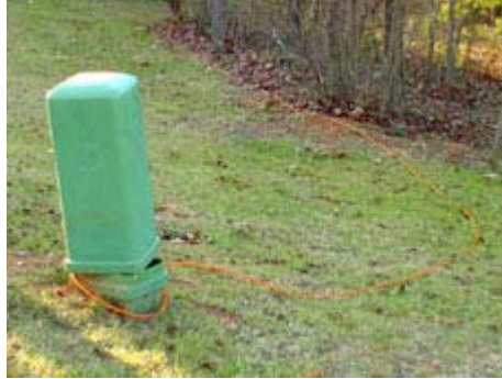
In this underground code violation, cable-tv pedestal lid and coaxial cable lie on the ground rather than under it.
