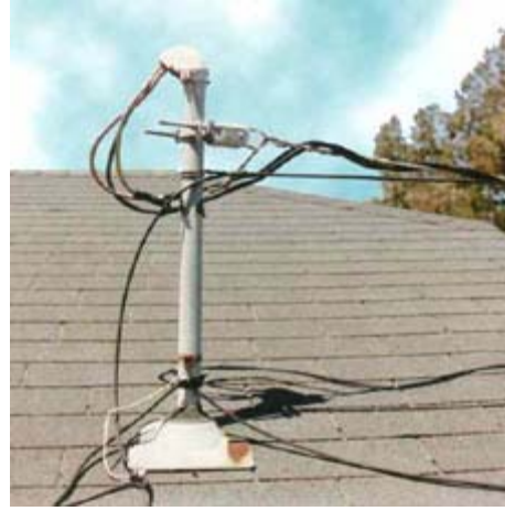
Here, the cable code violation is a cable-TV drop touching a power drop.
