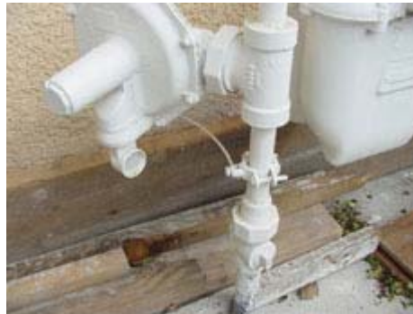
Here, the cable-TV system also is grounded to the natural-gas meter pipe.
