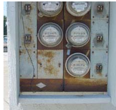
In this grounding violation, the cable-TV system wire is undersized and blocks meter panel access.
