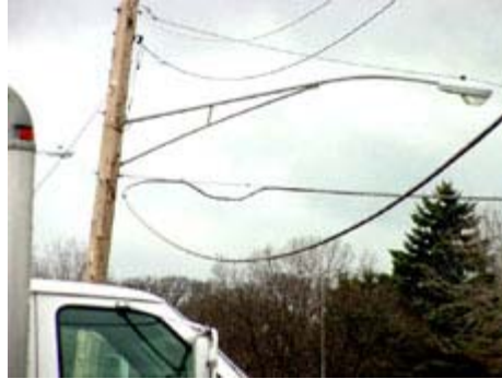
This cable-TV system hangs too low over a roadway.
